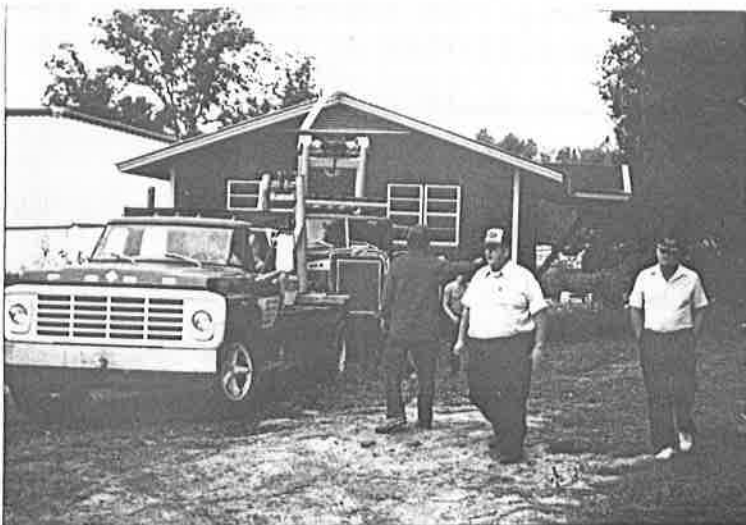
MR. FAUVER WITH HIS MEN AND LLOYD WITH TWO TRUCKS PULLING THE HOUSE FROM IT'S OLD LOCATION ON AIRPORT AND UNIVERSITY BLVDS.
