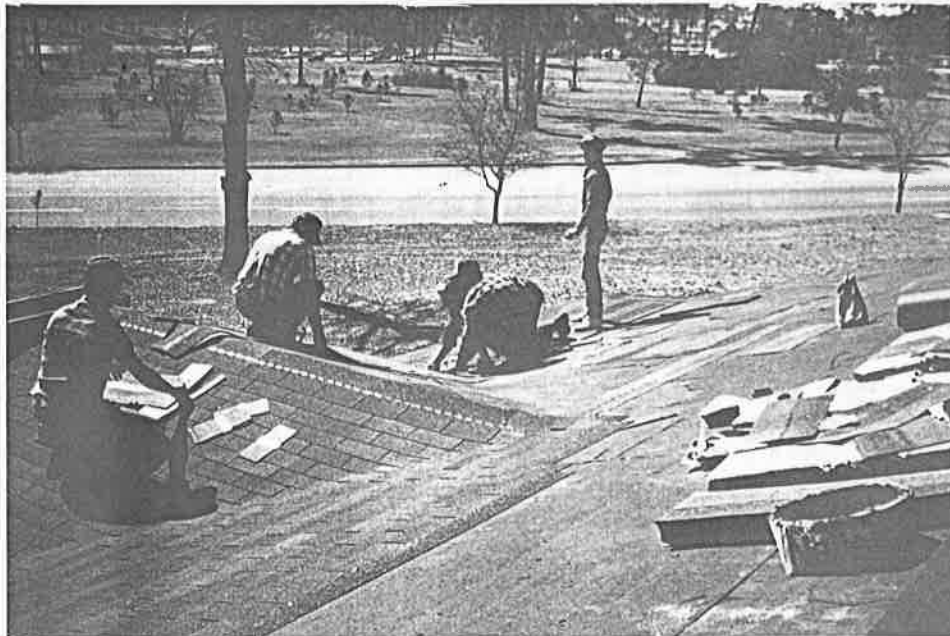
A GROUP OF OUR MEMBERS RE-ROOFING THE FRONT OF THE CLUB HOUSE WHILE CECIL'S SON-IN-LAW, RONALD GRIFFIN, WEAVES SHINGLES IN A VALLEY.
