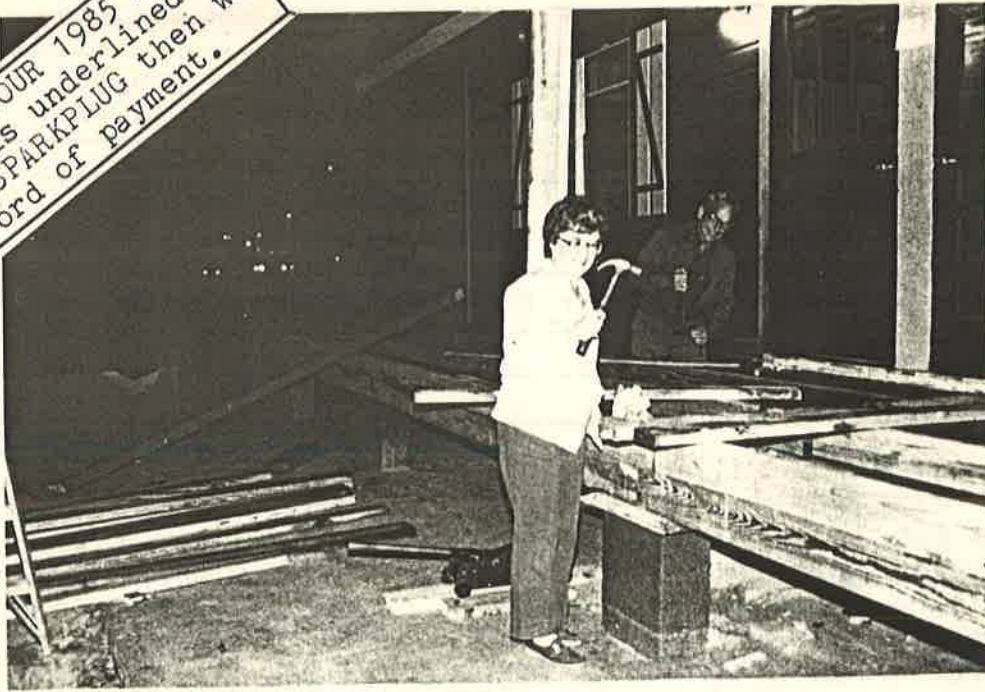
THE DSR's FIRST LADY, LYCYLE CROWDUS, SWINGS A MEAN HAMMER BUILDING THE CLUB-HOUSE PORCH!
